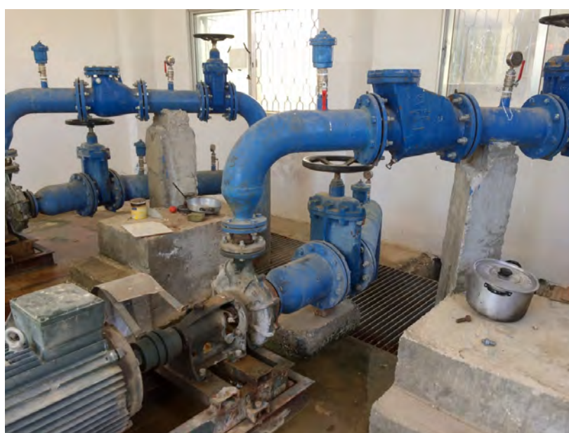
Figure 23: Leaks at ground water pumping station in Ma'an
