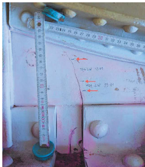
Figure 4: Crack caused by dynamic load
