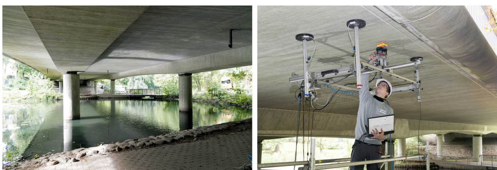
FIGURE 1 Photos of the investigated bridge (left) and of the mounted structure scanner equipped with a GPR antenna (right; extracted from (Maack, Küttenbaum, Epple, & Aligholizadeh, 2021) 8 )
