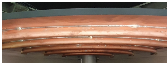
Figure B.3 Copper thermofluid pipes
