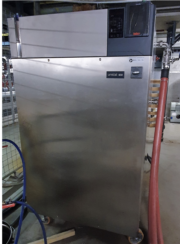
Figure B.4 Process Cooling Unit
