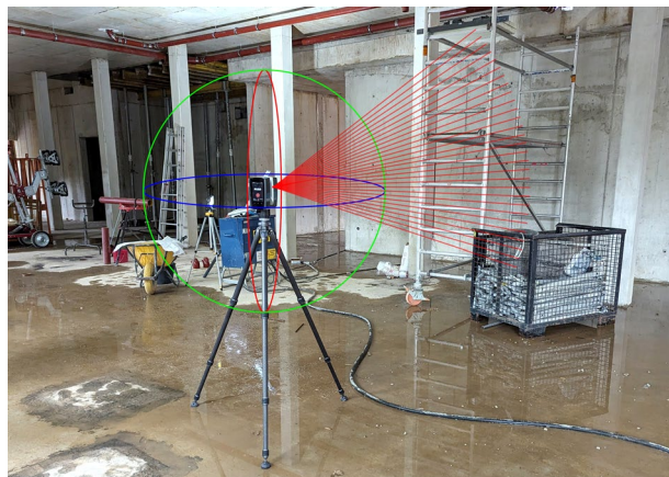
Fig. 2 Exemplary illustration of the terrestrial laser scanner device that was used to record the data. The laser scans the room in a spherical grid. The scene in the background shows an example of a particularly challenging situation on the construction site, which presents difficulties for the optical measurement method due to the confusing scene, the building materials, tools and temporary support structures stored on the construction site, and puddles of water on the ground, which irritate the laser reflection.
