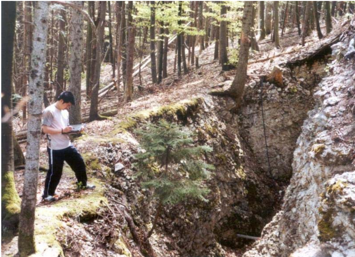
Figure 51: The landslide area near Balingen in Germany
