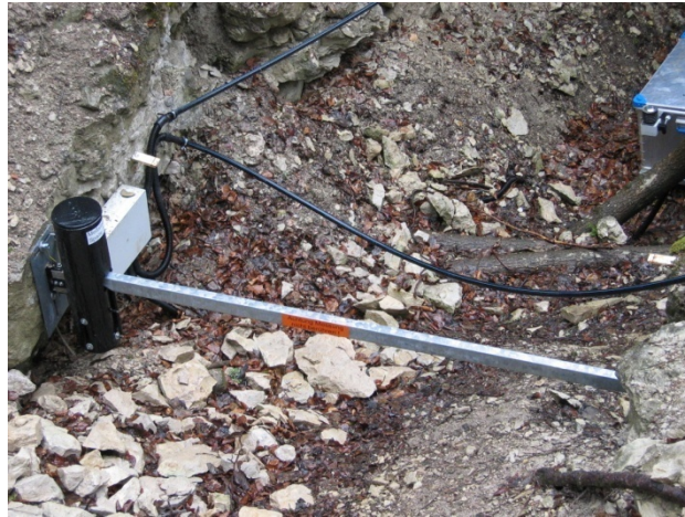
Figure 66: Extensometer monitoring a Ditch.
