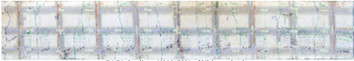
B1C1, loading 60kN, 79% of Ultimate load
